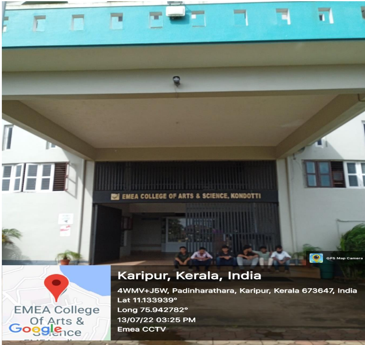
CCTV Camera at Main Entrance
