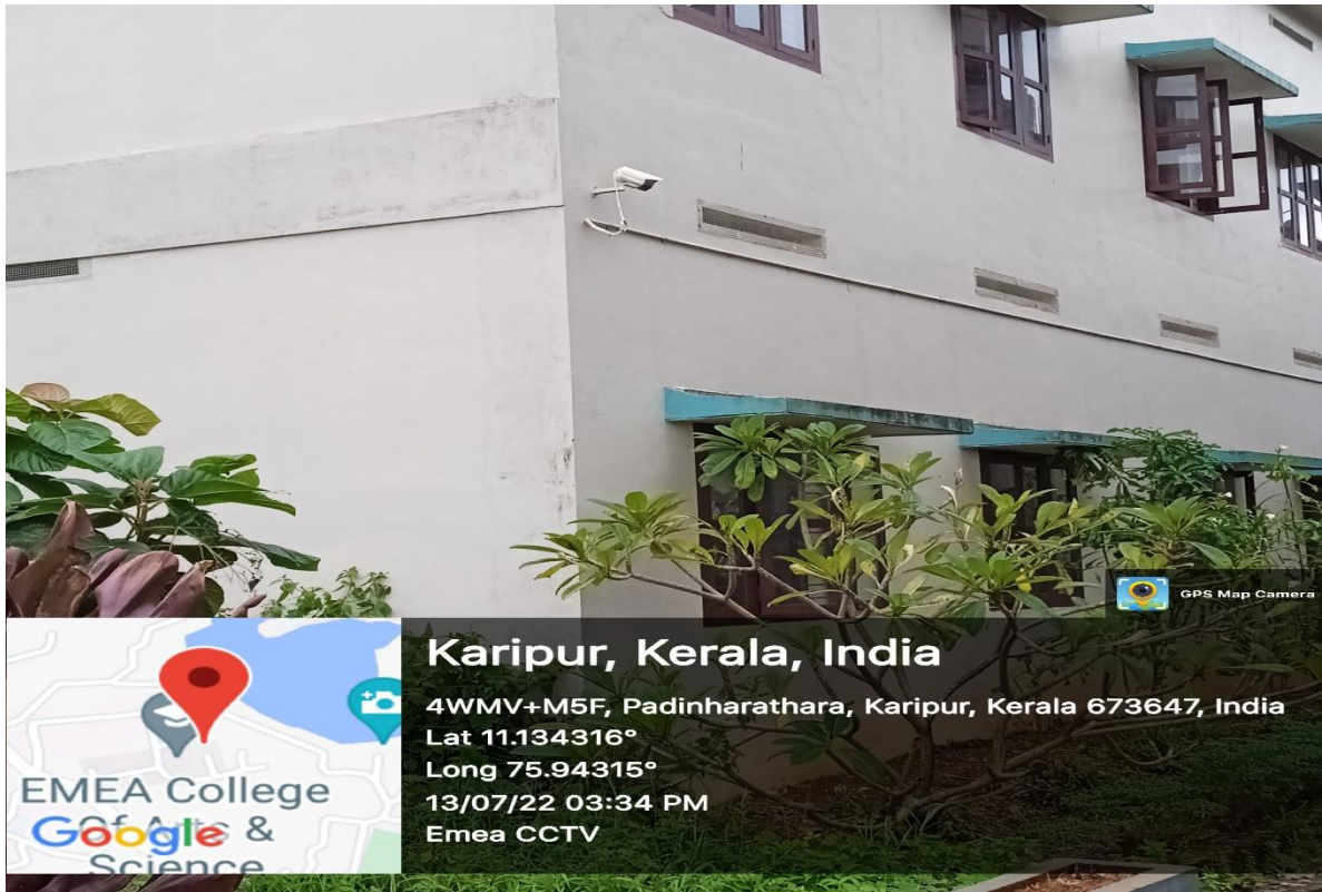
CCTV Camera at front side of main block
